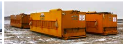
4 of 6 - Blow Back Tank
